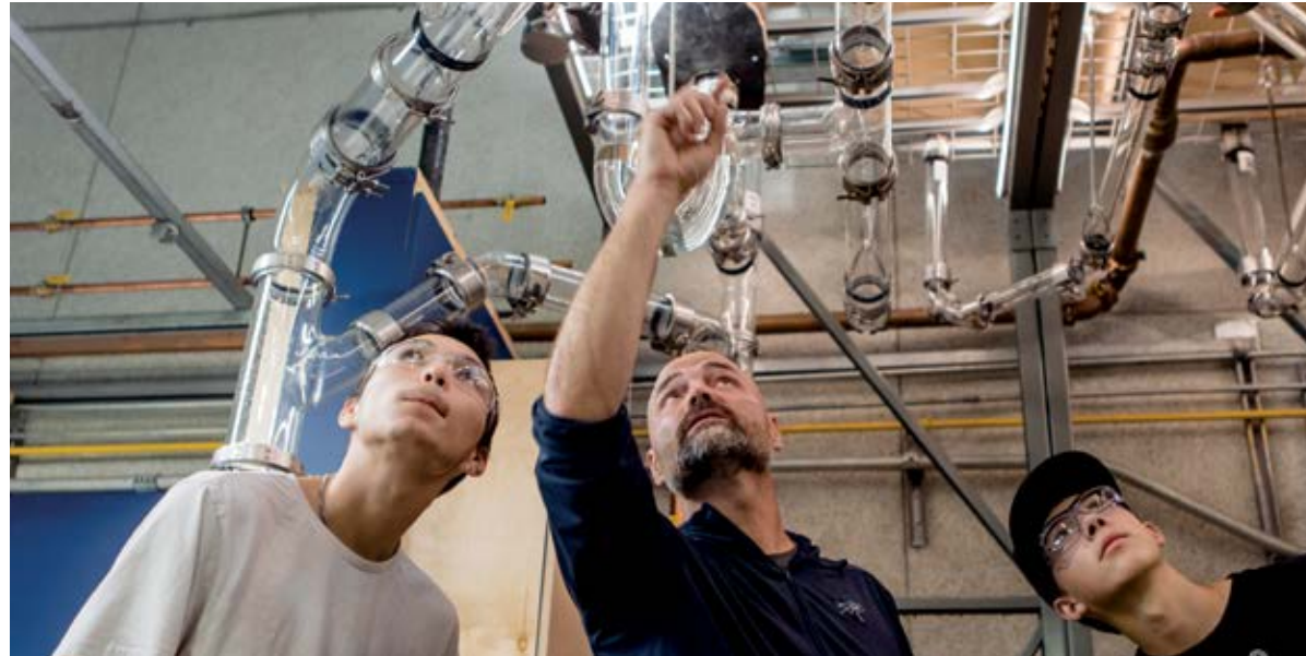
Associate Professor Paul Simpson shows two young students how a multi-piping system works.
